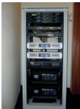
KV2 and QSC amplifiers racked with Furman FS-Pro E series II power conditioners
